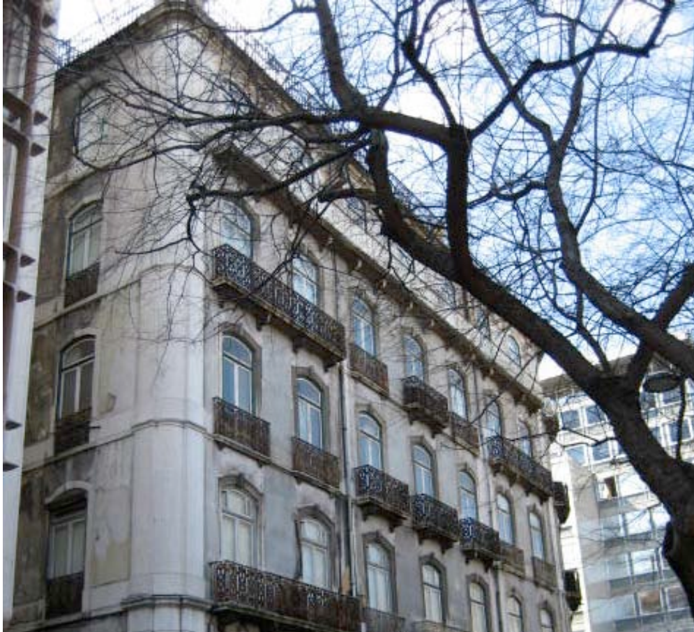
Another picture of the abandoned building in Avenida Liberdade 195-211 in Lisbon
